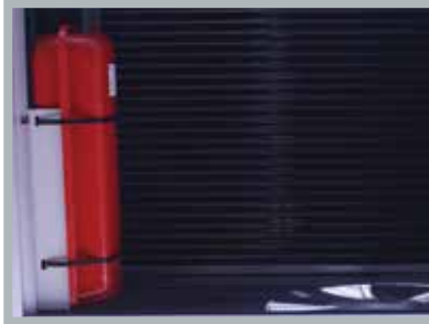
closed expansion tank
