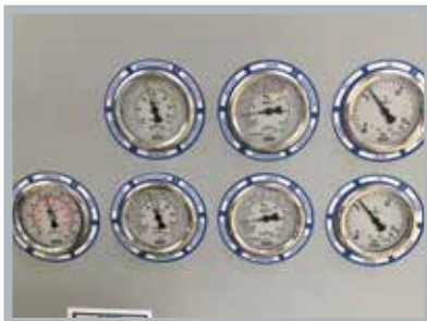
refrigerant and oil gauges
