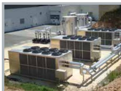
high capacity process chillers
