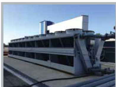
free cooling chillers
